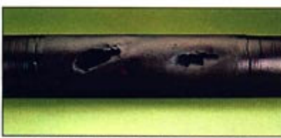
▲ HOLES ON EXISTING PIPELINE →
