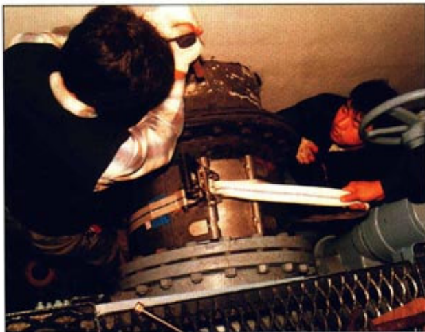
▲ VIEW OF INSTALLING A REPAIR CLAMP(RC-L) ON 500mm DIAMETER PIPE WITH SPECIAL BELT
