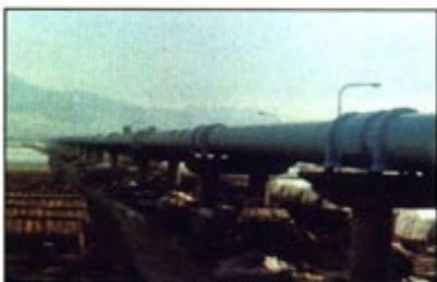
▲ ABOVE-GROUND LINE FOR LARGE WATER SUPPLY PIPELINES
