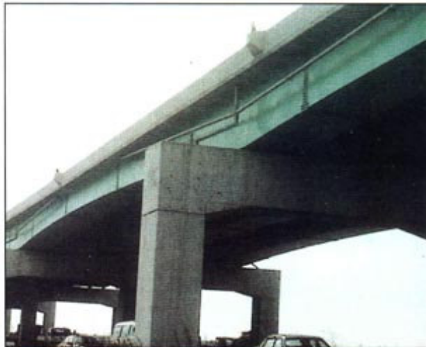
▲ DRAIN PIPELINES ON LARGE BRIDGE FOR VIBRATION-PROOF
